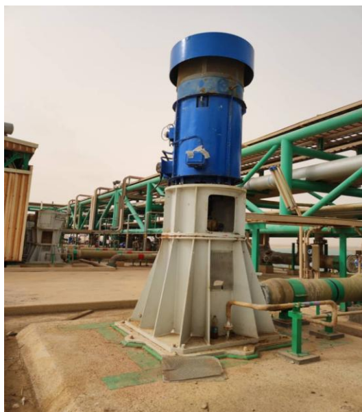
Fig. 9. Sea Water Intake Pump
