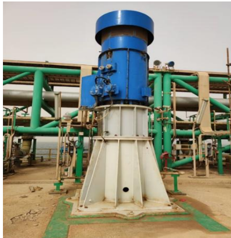
Fig. 18. Sea Water Intake Pump
